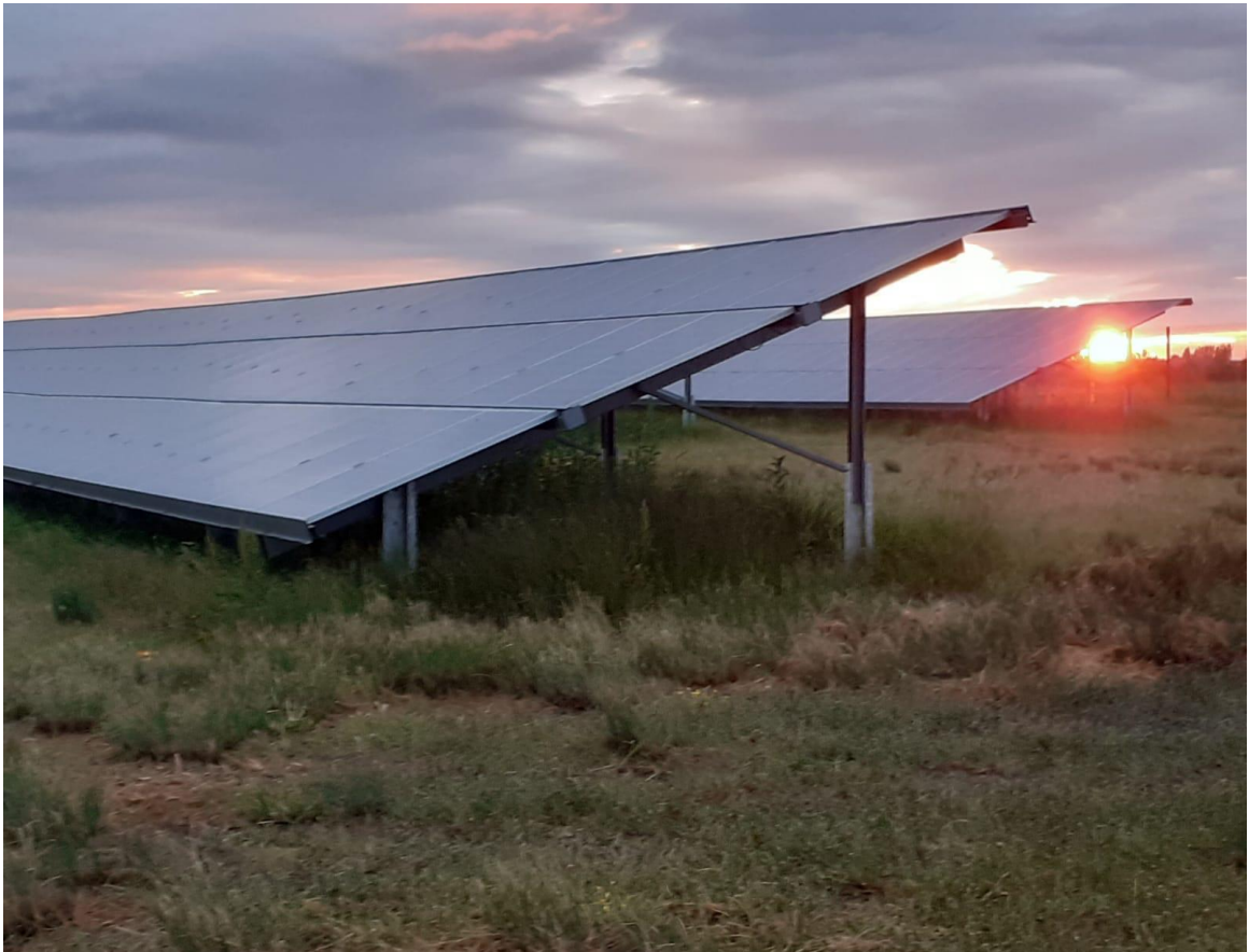
Photo Solar Farm at the former Gedling Colliery
